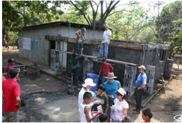
Belen construction; team is also distributing books to be used by local community.
